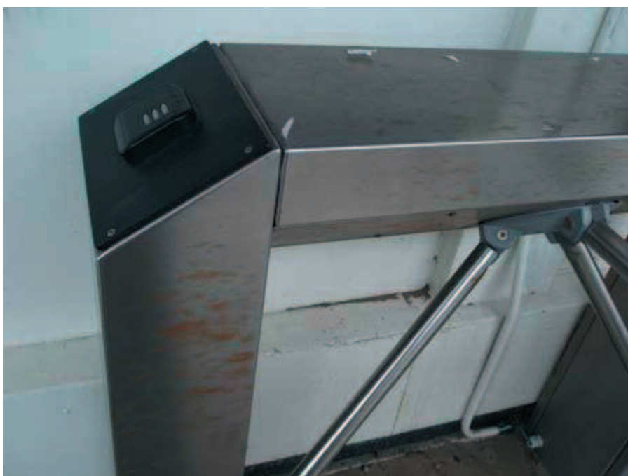
Fig. 2. RVS 316 access gate corroded by aerosols.
