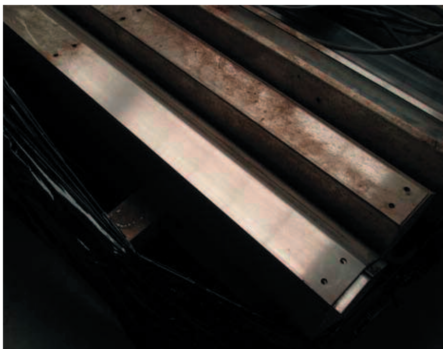
Fig. 4. Contamination corrosion on 316L light fittings (the bottom fitting has partially been treated with the organic acid Innosoft B570).
